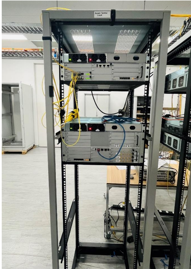
Master Unit Site at two central locations
