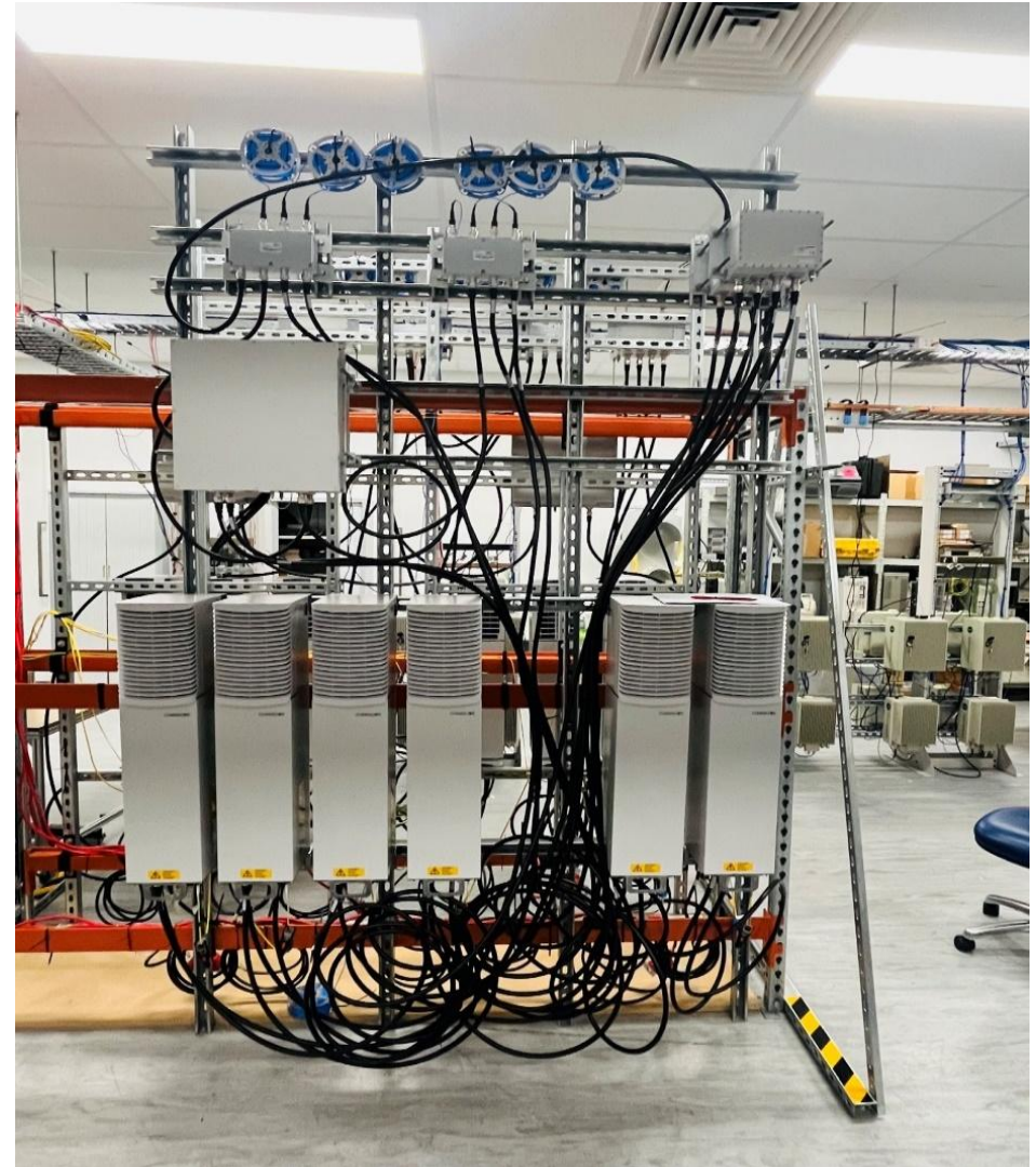
Remote Unit Site in tunnel and every station
